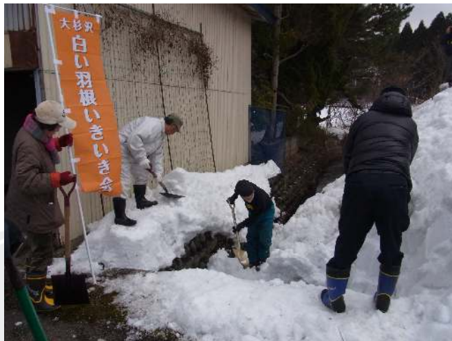
Snow Removal of inside of the drain
