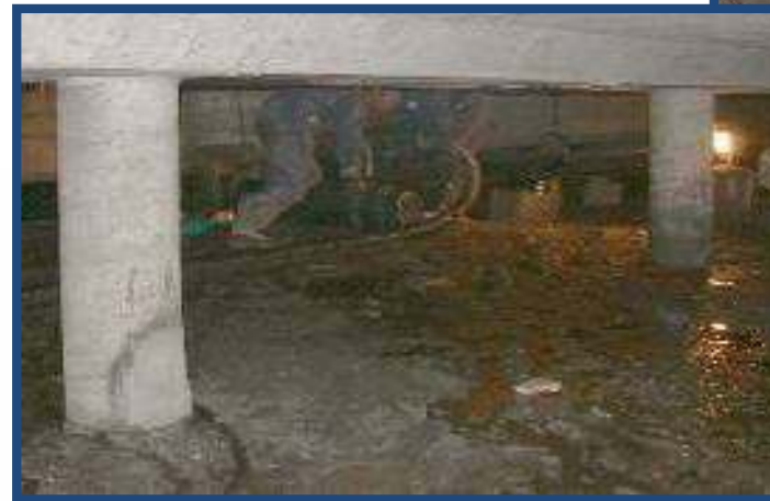
Mud Pumping in structural elements
