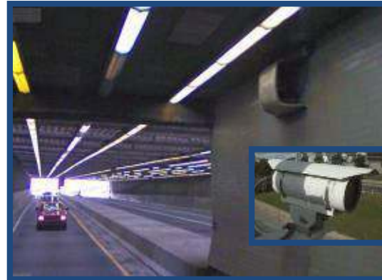
Camera in climate-control housing
