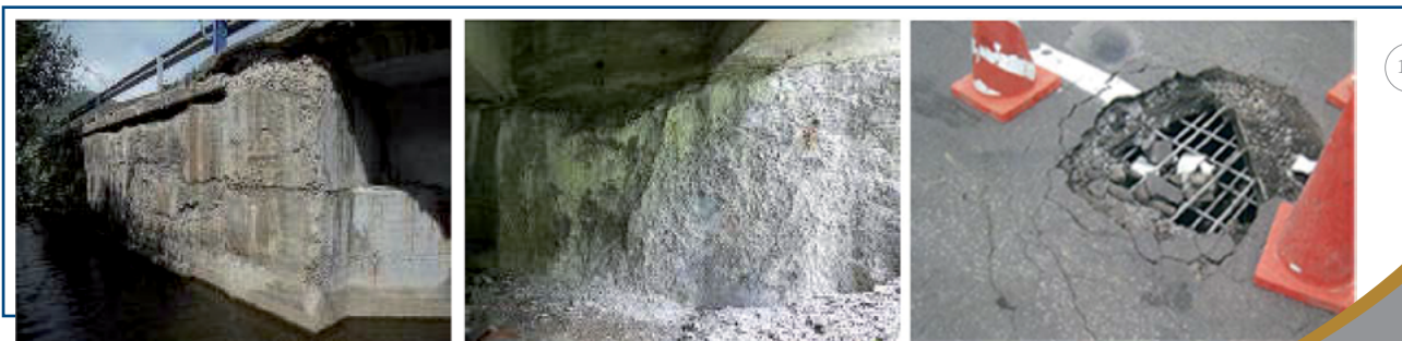
Illustration 15 (theme 8) - Damage at abutment, sidewall and surface due to freeze-thaw cycles
