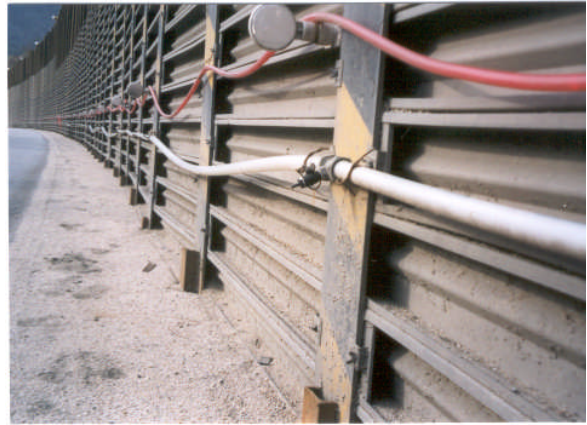
Figure 2 – Fixed de-icing spray system
