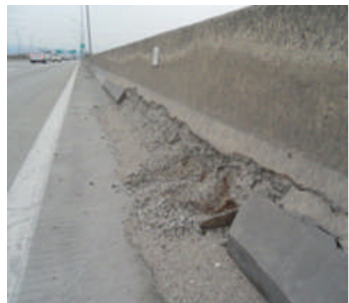
Figure 4 – Deterioration of barrier
