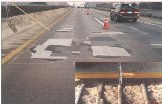
Figure 3 – Deterioration of deck
