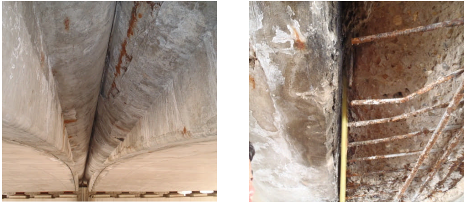
Figure 9 – Deterioration of deck under longitudinal joints
