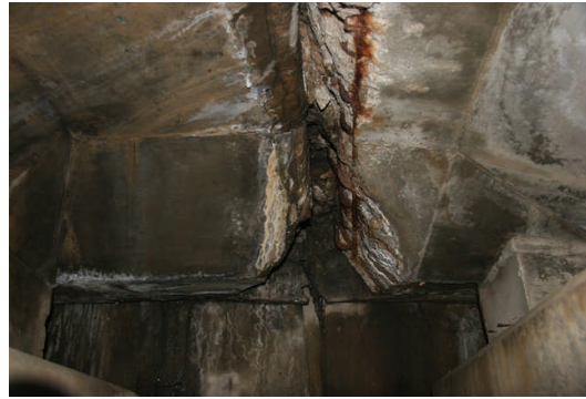
Figure 7 – Deterioration of decks
