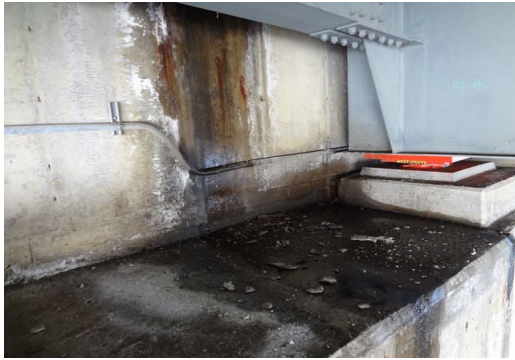
Figure 6 – Leaking expansion joint
