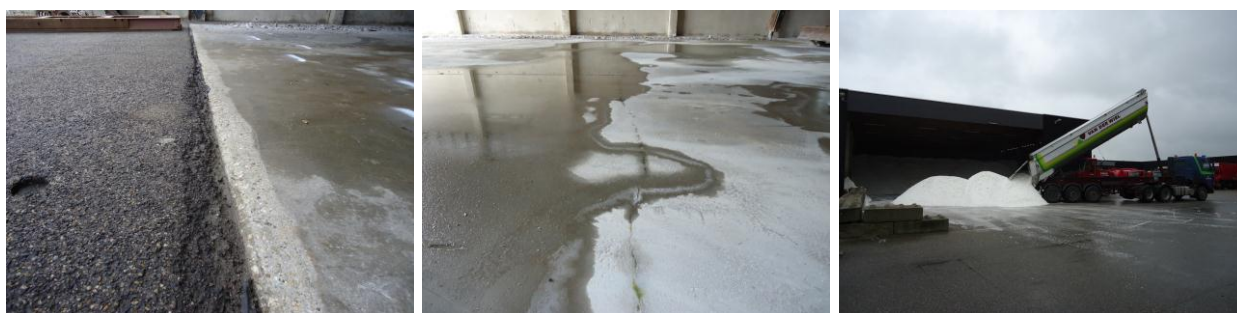
Figure 3 – Indoor salt storage and situations where water and brine can enter the soil
