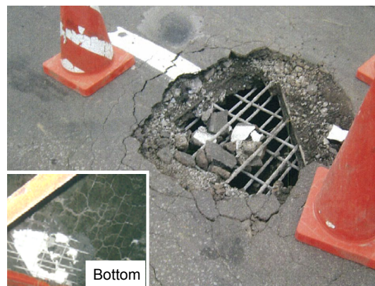
(b) Subsidence of RC slab
