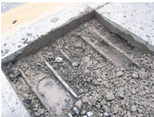
(a) Frost damage of cover concrete
