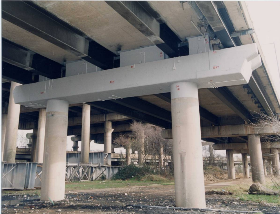
Figure 2 - Conductive Paint Anode Cathodic Protection System on typical Midland Links substructure.
