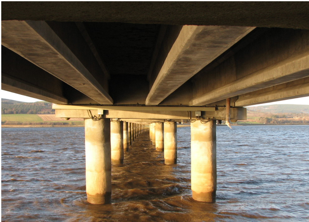
Figure 3 - MMO Coated Titanium Mesh Anode in Cementitious Overlay on Cromarty Viaduct Pier on the A9 in the north east of Scotland
