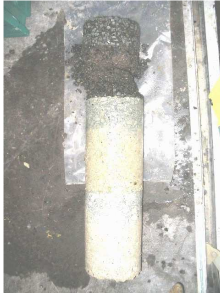
Figure 2: Core drilled near a pothole Disintegration of the old surface layers
