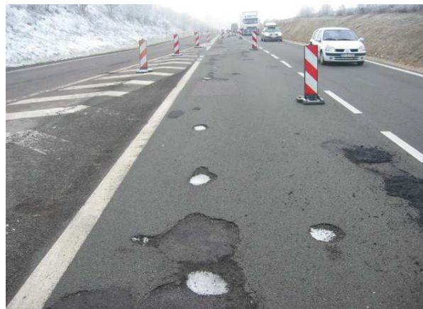
Figure 1: Series of potholes which appeared in a few hours
