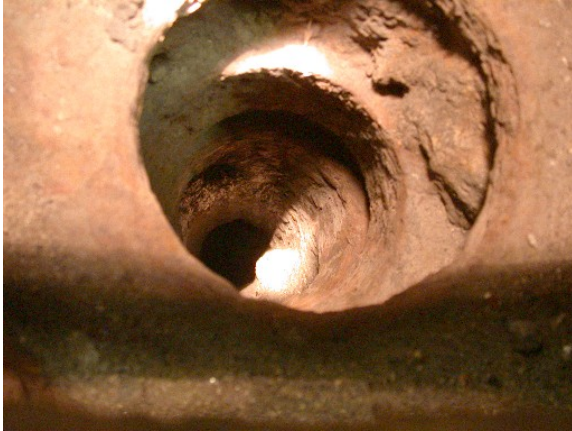
(a) 55% blocked drain
