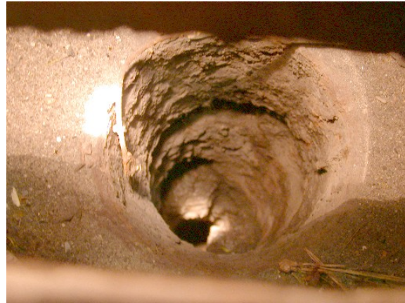
(b) 97% blocked drain
