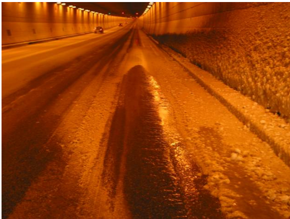
(a) Ice patches on pavement
