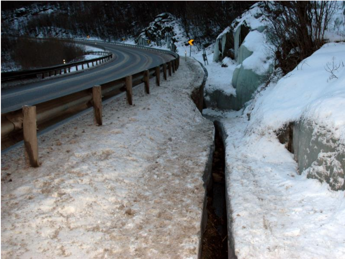
Picture 9 – thawed ice cut leading to culvert from both sides along national road E6 Photo: Heatwork
