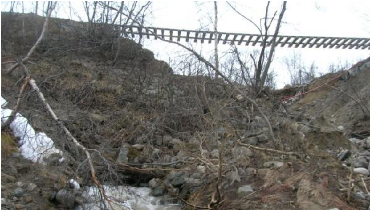
Picture 2 – Railway damage Photo: NNRA
