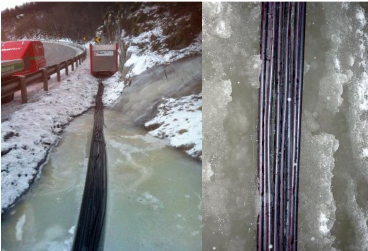
Picture 8 – Subcontractor thawing drain trench for NPRA (left). Bundle of eight heater hoses (right) Photo: Amarkussen AS
