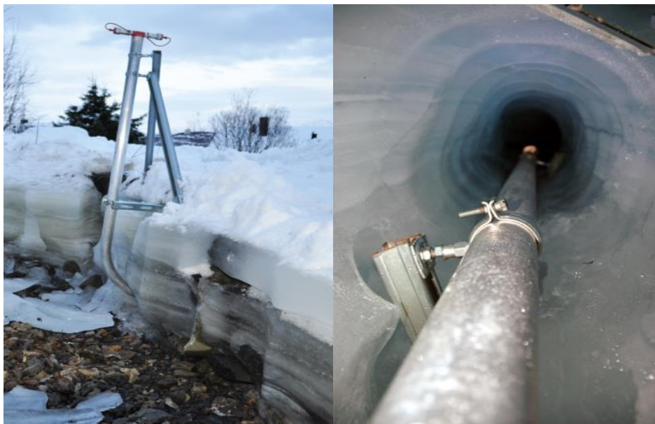
Picture 4 – IGS installed in frozen culvert (left). Excess water way through solid ice (right)
