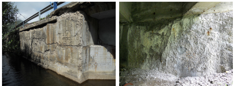
Figure 13. Damage at abutment and sidewall due to freeze-thaw cycles
