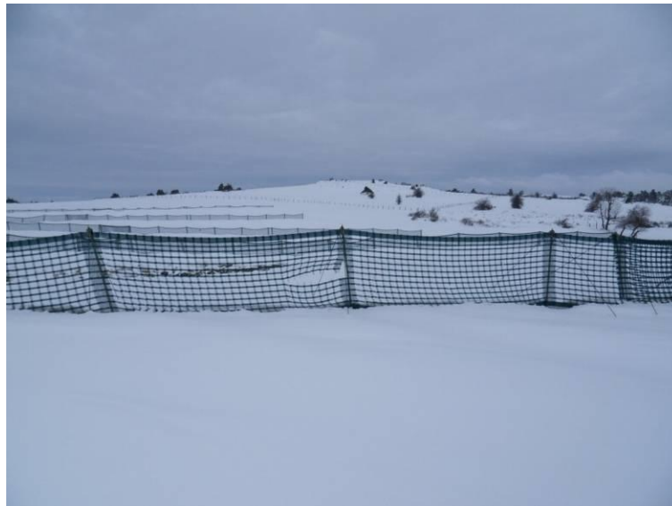
Photograph 6: Fences sag and tear when not adequately tensioned.
