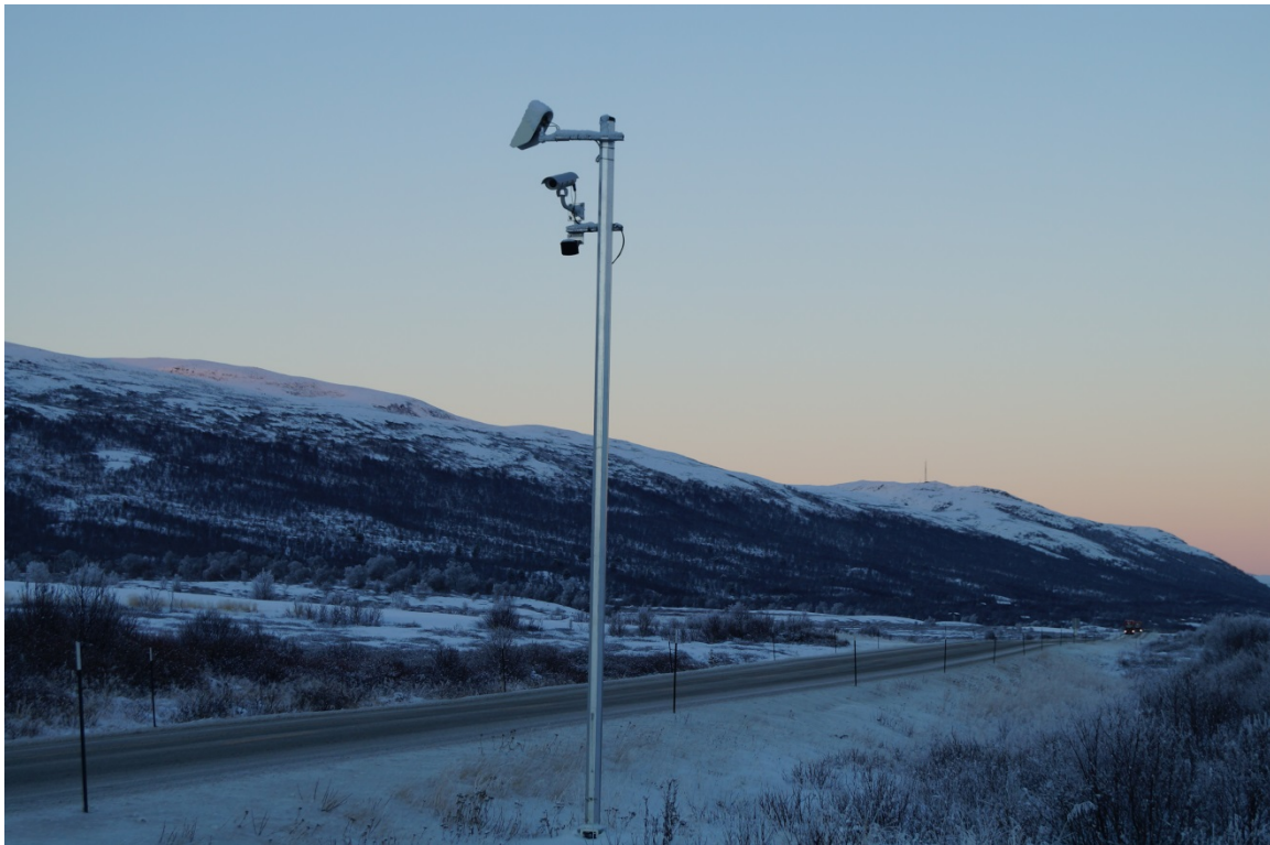
Figure 3 - Weather station with wind sensor, web camera, surface- and air temperature and a road surface state sensor.
