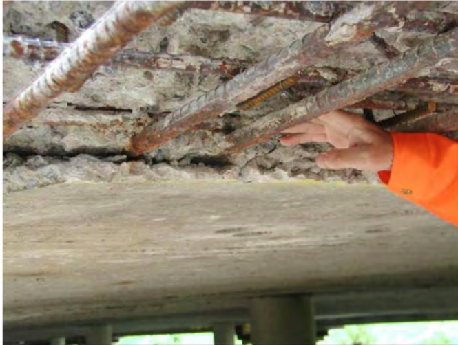
Fig. 1. A bridge deck subjected to de-icing salts.
