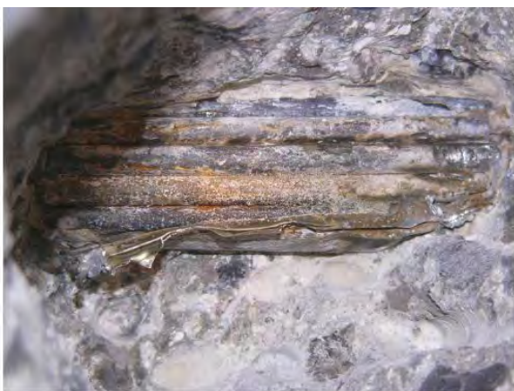
Fig 6. Corroded prestressed reinforcement due to chlorides.
