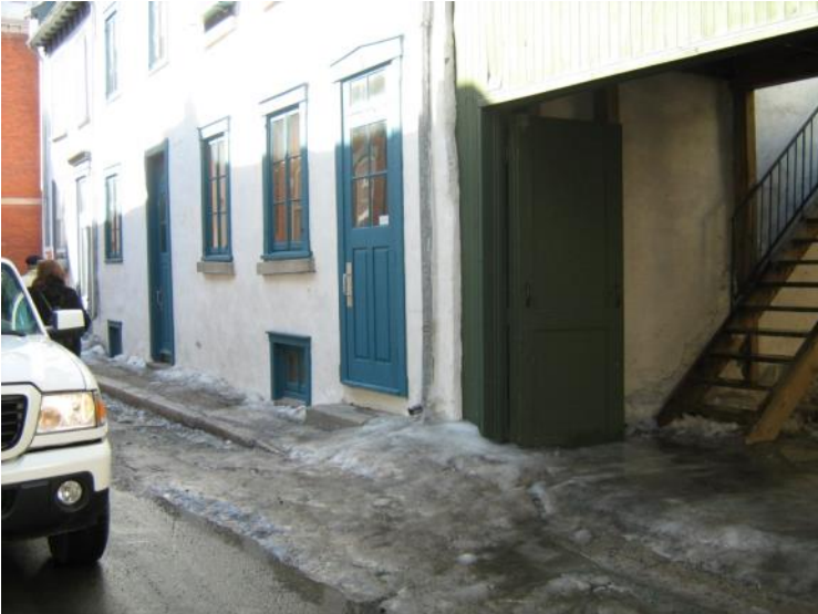
Photo 5 – Downspout draining directly onto the sidewalk
