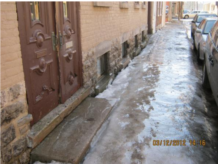
Photo 6 – Ice formed by water dripping from a roof onto the sidewalk
