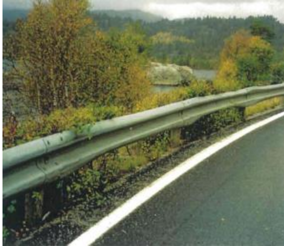
Figure 1: example of damages due to snow clearing operations
