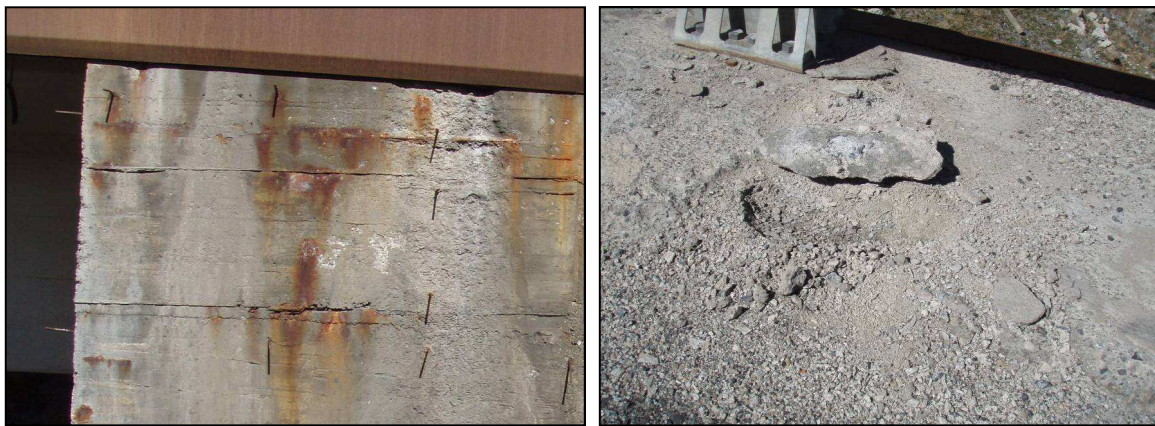
Figures nº 12 and nº 13. Degradation of concrete abutment No. 2 (left) and surface alteration of concrete base for safety barrier (right)
