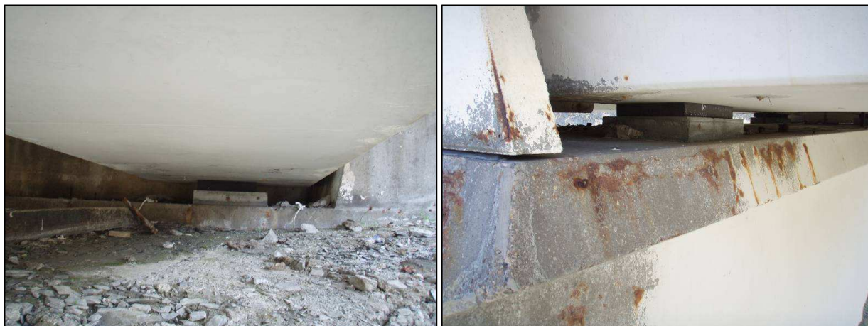
Figures nº 5 and nº 6. Left beam bearing at No. 1 abutment (left) and right beam bearing at pier No. 2 (right)
