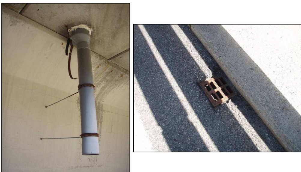
Figures nº 8 and nº 9. Drainage tube at No. 4 span (left) and sink at No. 2 span (right)
