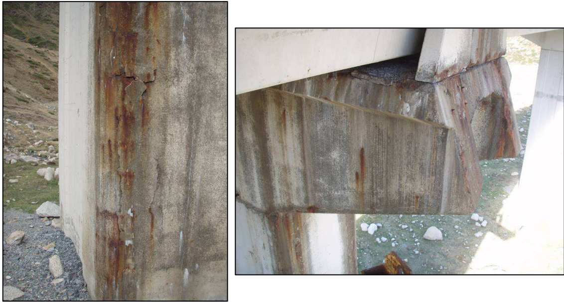
Figures nº 14 and nº 15. Detail views of spalling, stains and alteration of concrete surface at bottom of pier No. 2 (top left) and detail view of the pier cap (top right)
