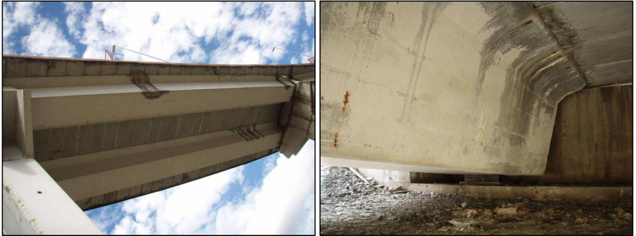
Figures nº 10 and nº 11. Concrete beams surface alteration with the presence of punctual reinforcements in sight
