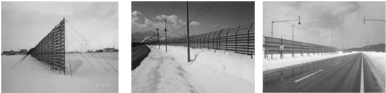
Figure 3 - Snow fences: traditional collector snow fence (left); collector snow fence (center); blower snow fence (right)
