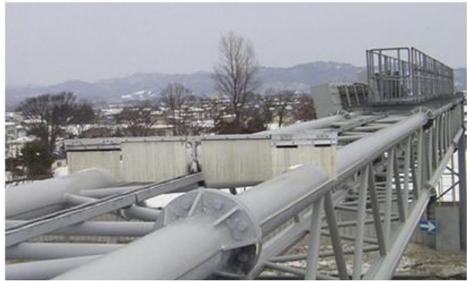
Photo 6: Installation conditions for Snow Clearing Device
